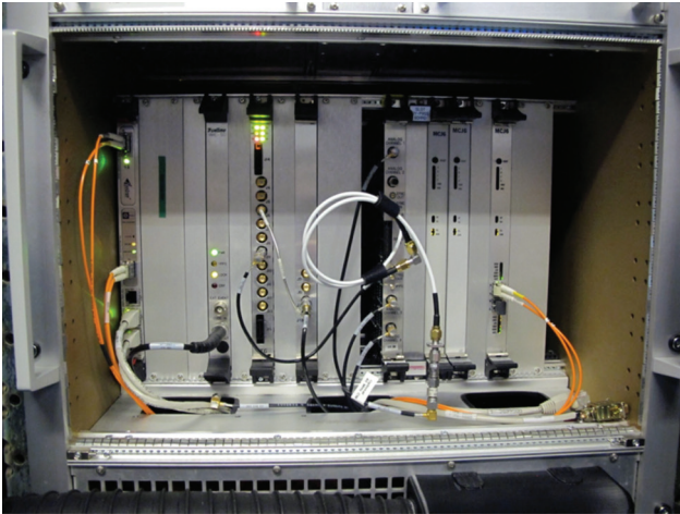
FIGURE 15. A ROSA subsystem consists of a VME chassis and a number of boards. Each subsystem, regardless of purpose, has a set of common boards, such as the VME controller, reflective memory board, and timing generator boards. Additional boards are added to perform the functions required. For the DPCS, Mercury Computer Systems DSP boards are installed to perform digital downconversion and pulse compression.
