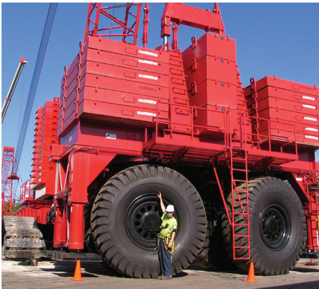
FIGURE 12. The author stands behind the auxiliary counterweight cart while a smaller crane assists with assembling the crane.
