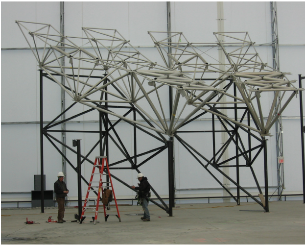
FIGURE 26. The first two radial rib sections are installed on their assembly stands inside the temporary building. Note the workers and the 8-foot stepladder for scale.
