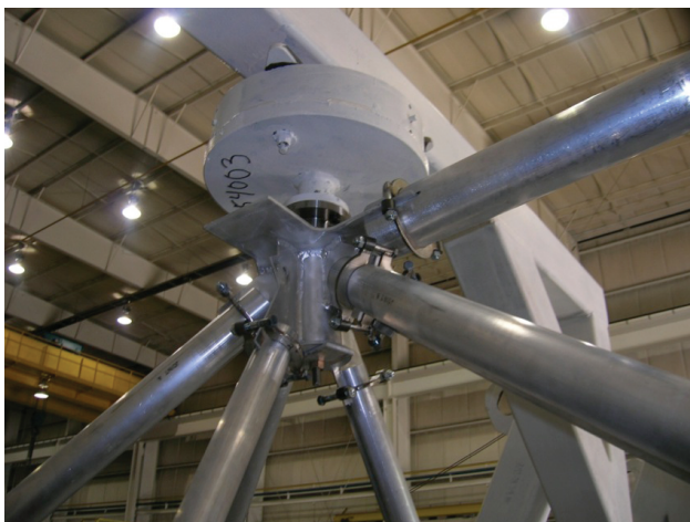
FIGURE A4. Fixturing of backstructure rib tubing to nodes prior to welding operations.
