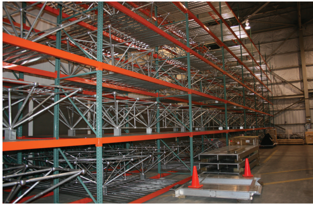
FIGURE 40. Completed subframe trusses await panel installation. All 104 subframe assemblies were stored on racks in an airplane hangar until they were transported to the site.
