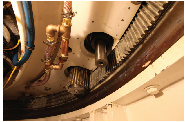
FIGURE 18. One of four pairs of pinions that drive against the stationary 12-foot-diameter bull gear. The shaft on the right is awaiting installation of the pinion gear.
