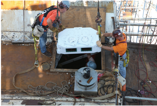
FIGURE 17. The first of the 1-ton gearboxes is lowered into the yoke. The gearbox was then transferred to a series of overhead chainfalls and a rail system in order to position it in place.
