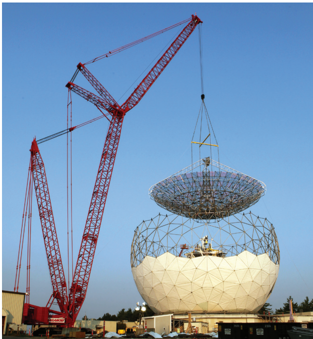
FIGURE 32. The new backstructure is carefully lowered into position on top of the waiting transition structure.
