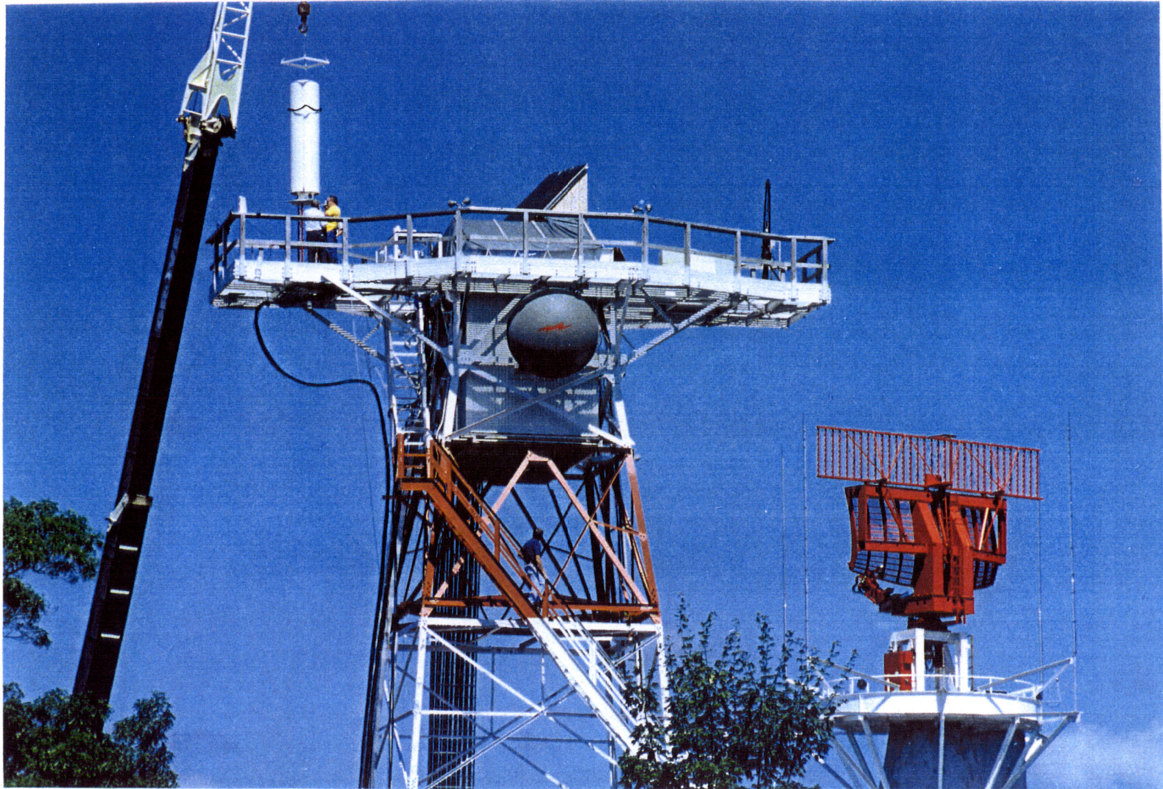
Figure 8. The antenna being mounted on the 70-foot lattice tower adjacent to the MODSEF Mode S Sensor.
