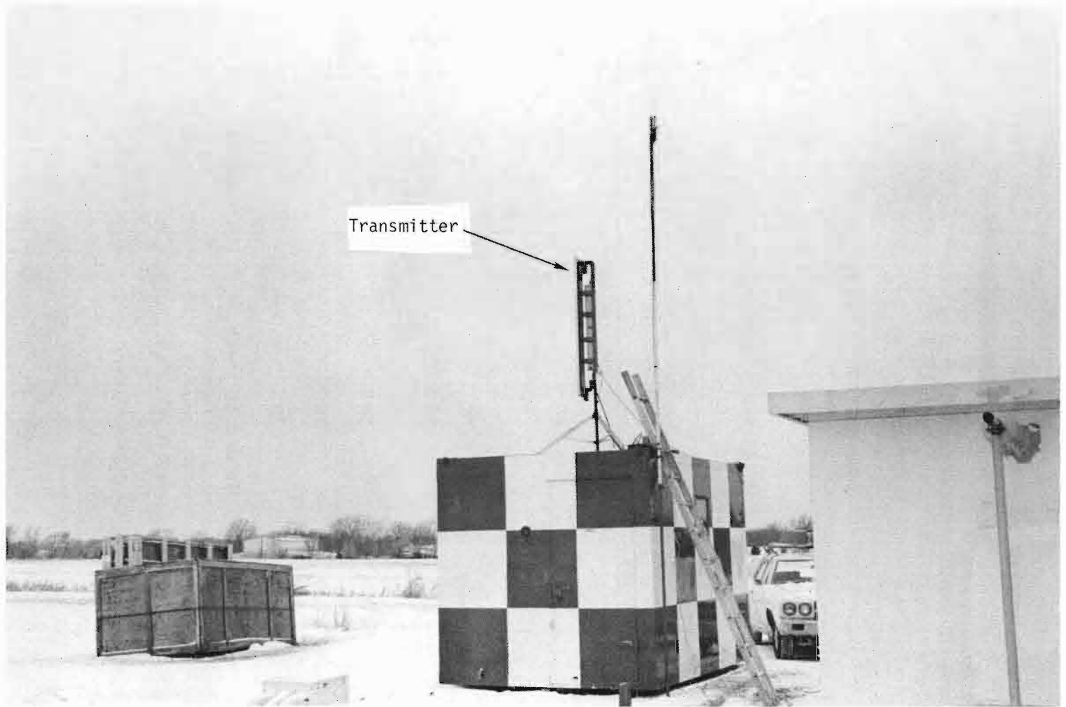
Fig. 3-62. Transmitter on localizer shack.
