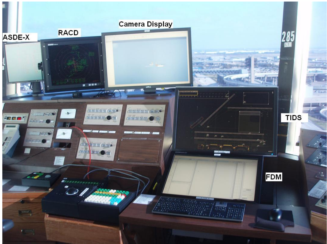
Figure 2-1: DFW-2 controller workstation
