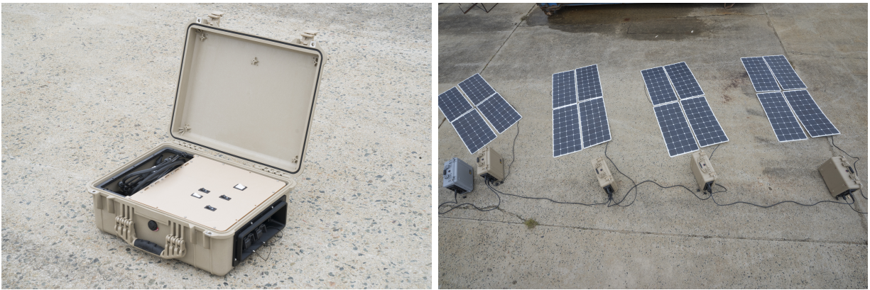
Figure 10. Inverter enclosure with cables stowed and multiple inverters setup for test.
